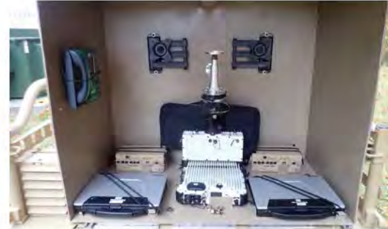
COMS Equipment Secured in the Enclosure
